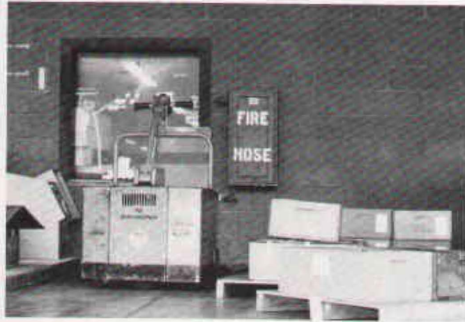
blocked firefighting equipment ...
