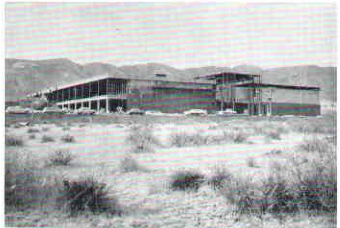
Two recent fires at construction site of new Colorado Springs plant are not expected to delay completion this summer.
